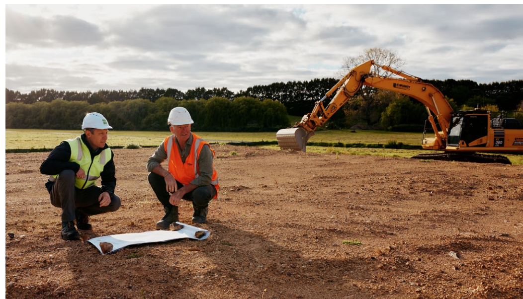
↗ Pictured left to right, Ben Shaw, Goodman Senior Project and Civil Manager and Gary Mundy, Managing Director G. Mundy Construction reviewing ground conditions at Waitomokia in Māngere, ahead of infrastructure works commencing.
