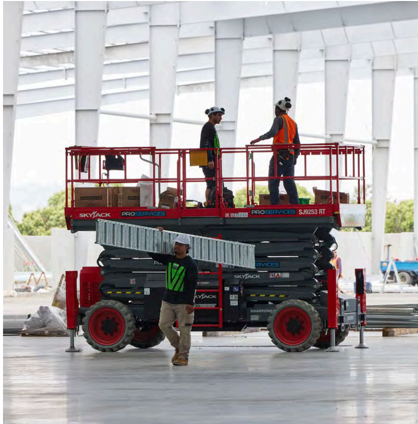
➤ Mainfreight supersite facility under construction at Favona Road Estate. The development is part of the $461.6m of active projects currently in progress.
